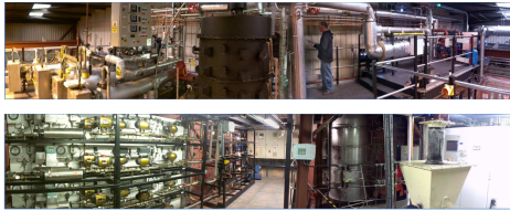
Panoramic photos of the 250 kW Combustion Test Facility
